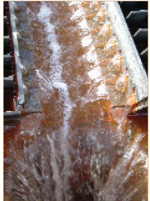
Water leaves a clarifier.
